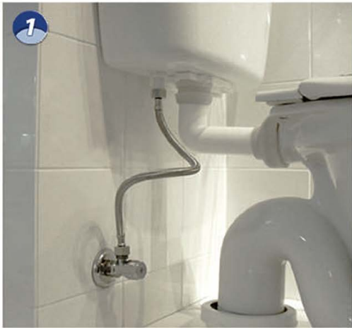
1 Most toilets have a flex pipe.
